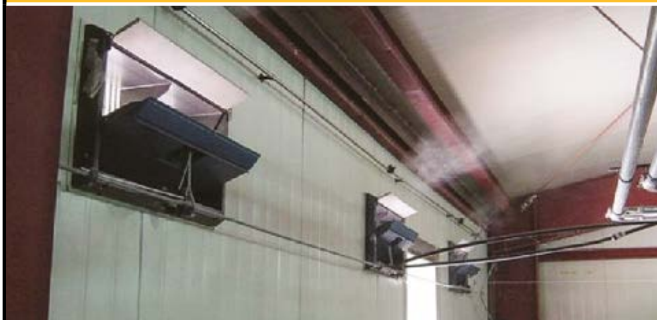
Figure 6.25 Example fogging system for a cross-ventilated house.
