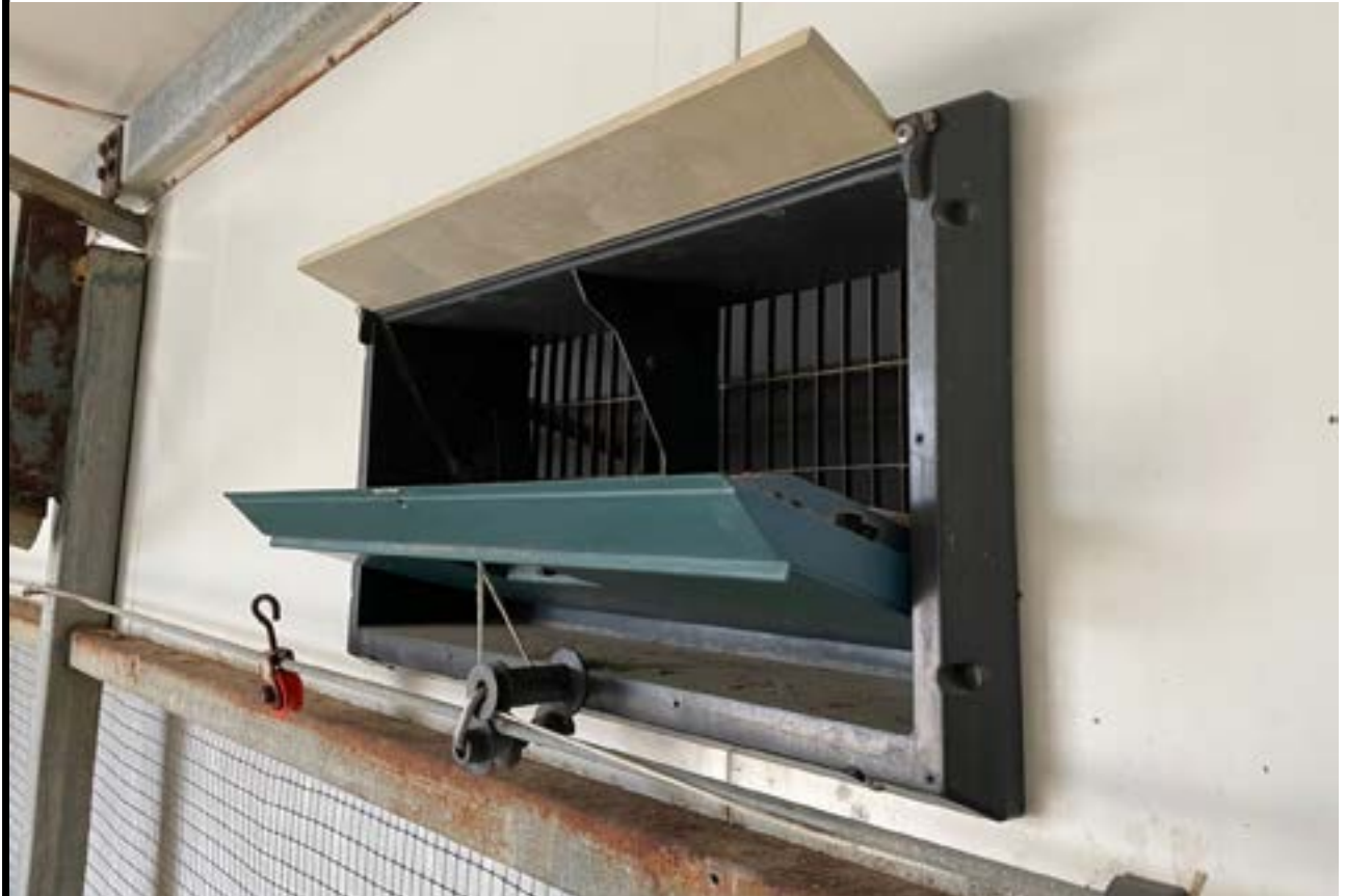
Figure 6.10 Example of a good-quality air inlet.
