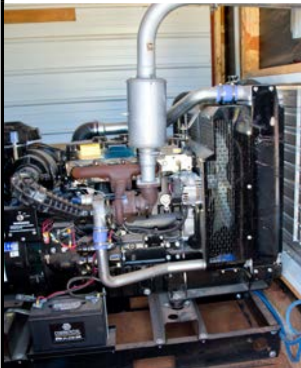
Figure 6.2 Example of a backup generator.
